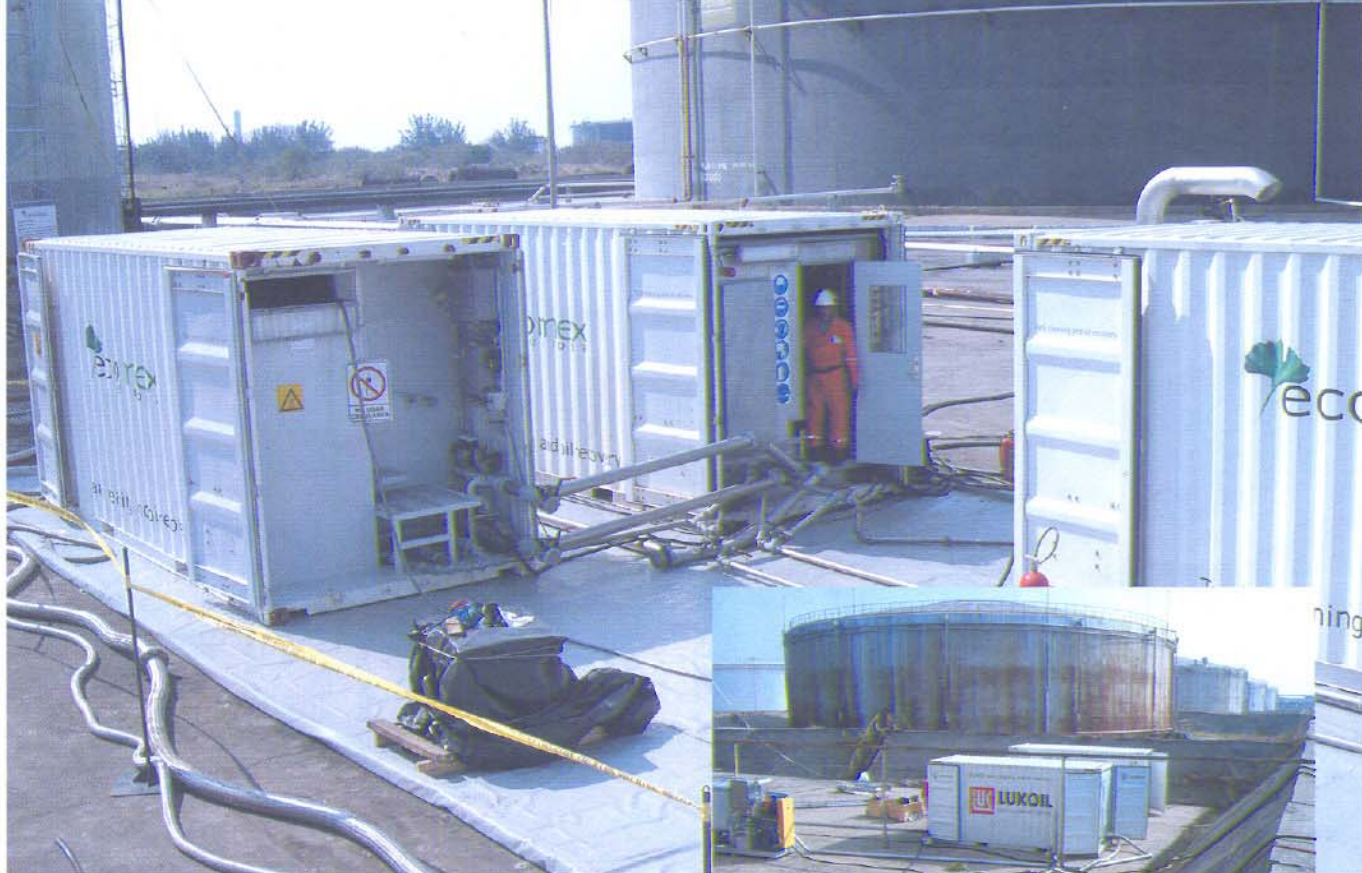
Figure 1. The BLABO system is in action at a site in Mexico. Oreco's BLABO system is a non-man entry solution. Here the BLABO system is in action at a site in Mexico.
