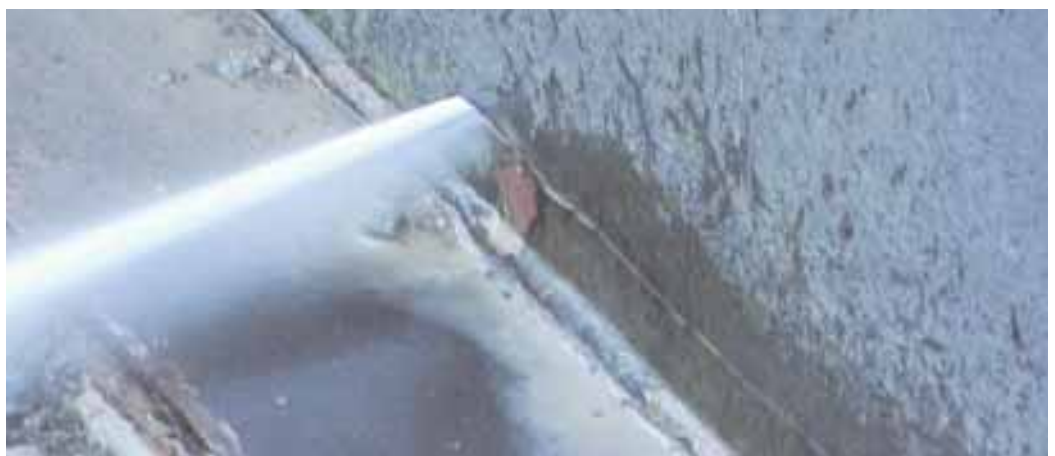
Cutting jet passing through the tank
